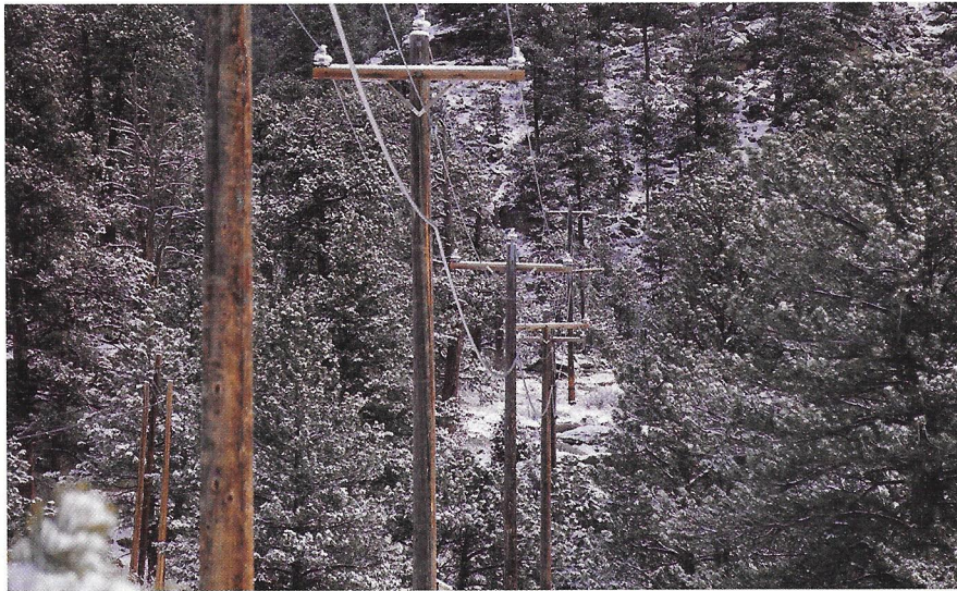
Due to the rugged terrain, only 40 percent of the area's utility poles are accessible.
